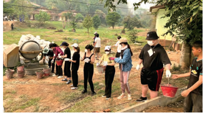
Cement Bucket Relay
